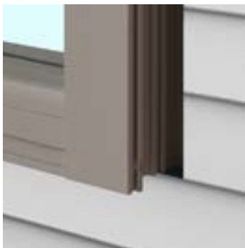
Window in weatherboard with no Flat Trim
