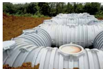
Drinking water storage (180m³). Stockage d'eau potable (180m³).
