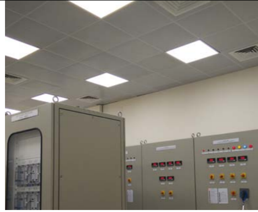
JEBEL SIFFAH SUBSTATION / OMAN
